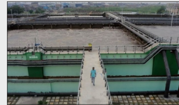
L & T, Ludhiana Project - CETP, Capacity - 40 MLD
